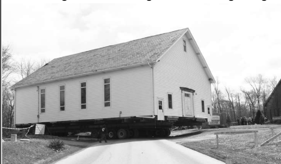
The 106-year-old Sonnenberg Church was pulled over the cribbing and planking, and across Hackett Road on a cold but partly sunny April morning. By noon, the church was positioned in the Sonnenberg Mennonite Church parking lot, ready to continue its journey westward through the woods, across the fields and to its permanent position in Sonnenberg Village where the structure will serve as the village's welcome center.
